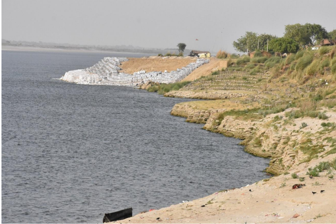
Image 31 : Use Of Sandbags For River Bank Protection Near Mahuli Ghat In Bhojpur
