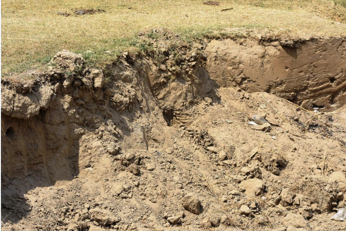
Image 32 : Bank Erosion As Observed Near Akauna In Bhojpur
