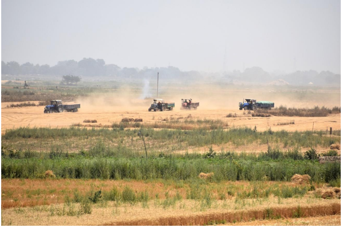
Image 33 : Rampant Illegal Sand Mining From Sone River Near Makhdumpur Village In Bhojpur
